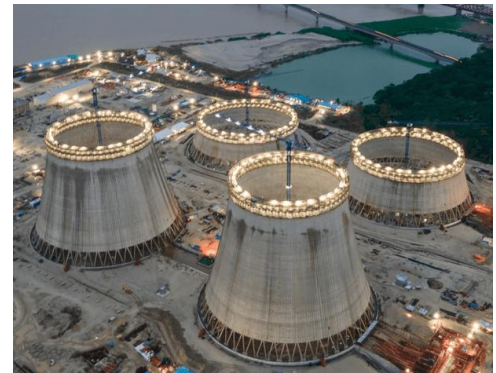
Picture: Cooling Towers of Power Unit 1&2
